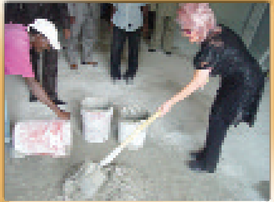
Jan pitched in and actually helped spread cement for the floor of the “Smile of a Child” hospital!
